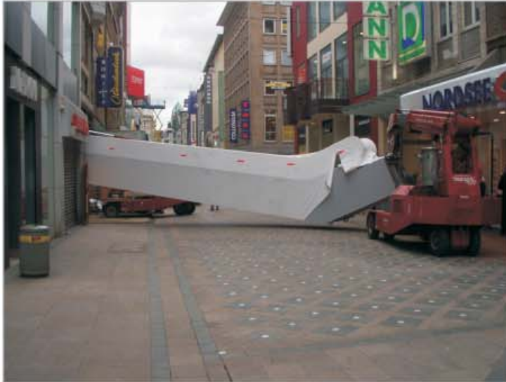
For moving-in the moving stairway the Westenhellweg had to be closed for a short-term.
